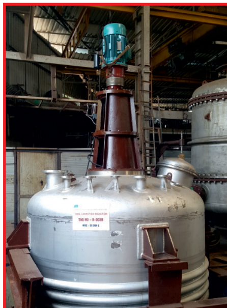
25 KL SS 904L Reactor
