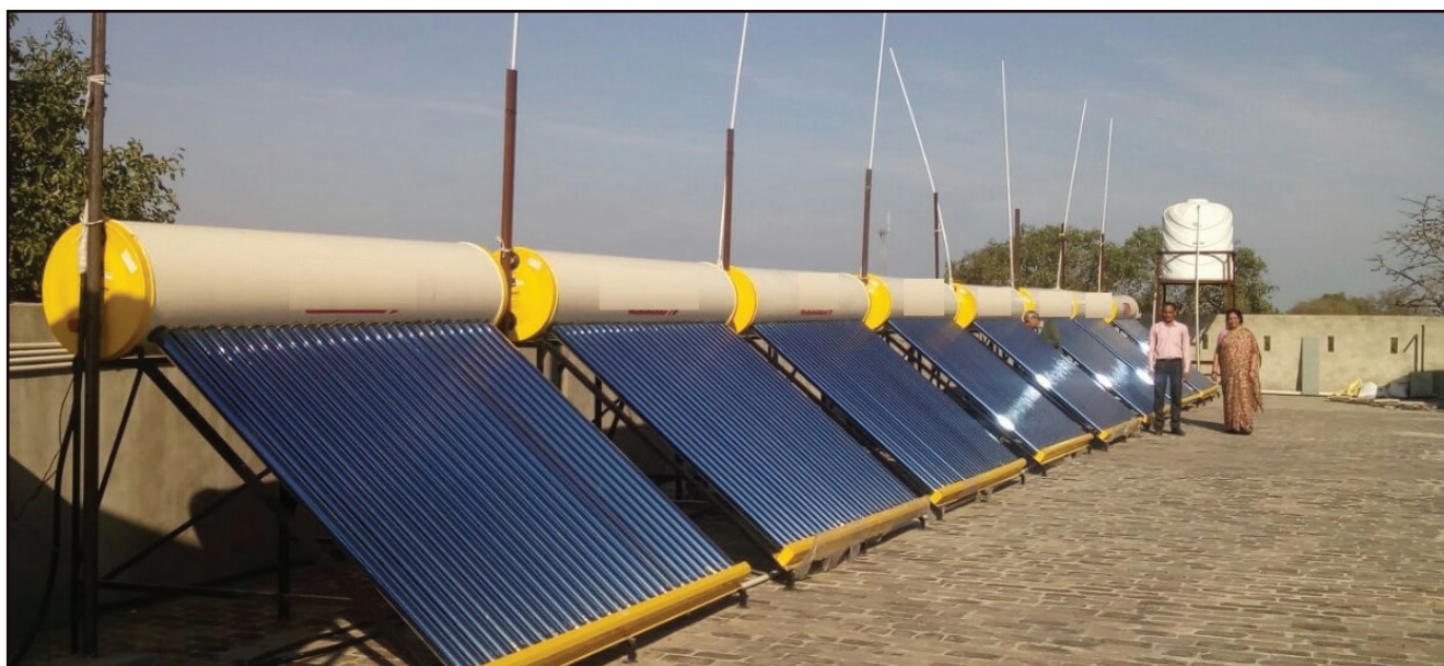
Solar Water Heater
