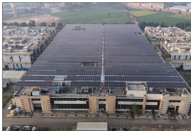
Roofsol Energy Project: Shriram Pistons & Rings Pvt. Ltd, Pathredi, Rajasthan, 1.9 MWp
