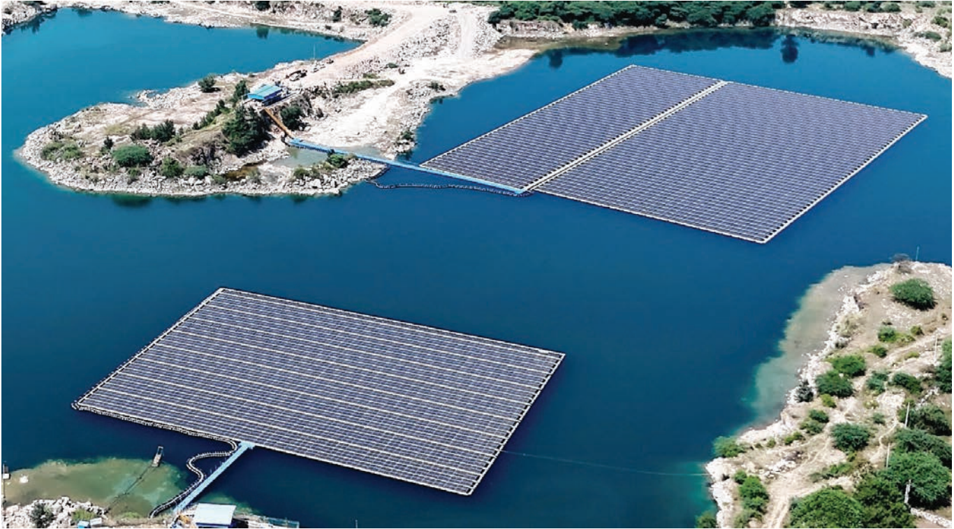
TrueRE's floating solar project, Udaipur, Rajasthan
