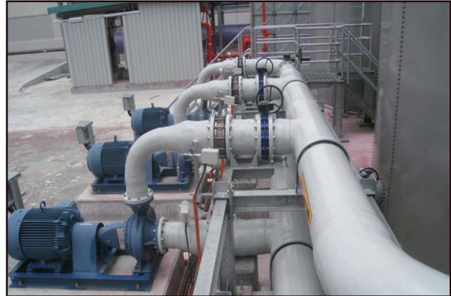
Changi NEWater plant in Singapore.
