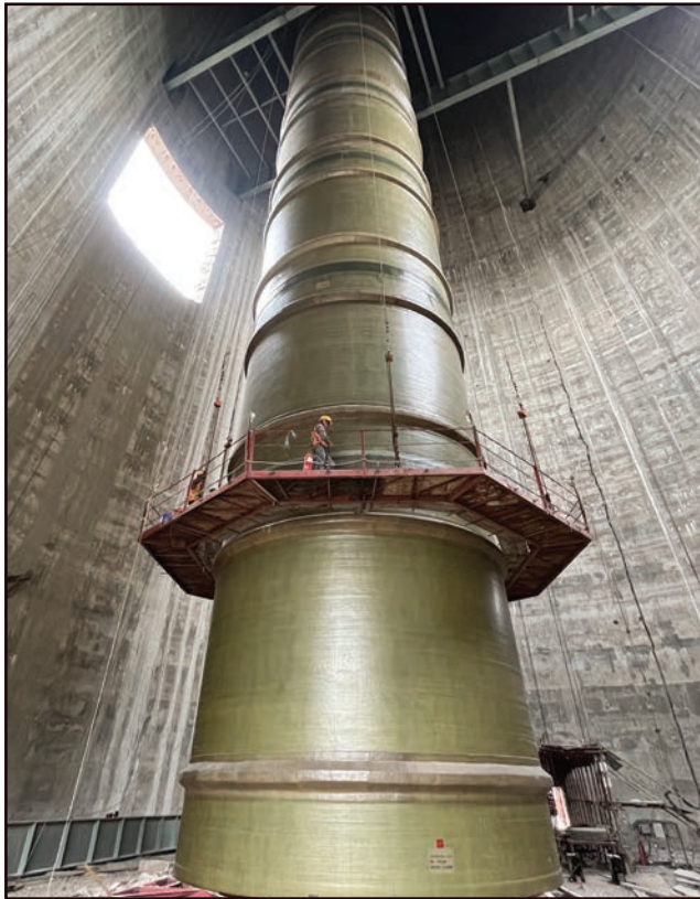
Project Maitree for BHEL in Bangladesh – transport of twin 7.6 meter diameter x 245 mt tall Stack liners.
