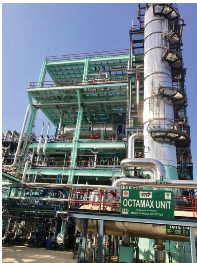
Fig. 2: 55 kTA Octamax® Unit at Mathura Refinery
