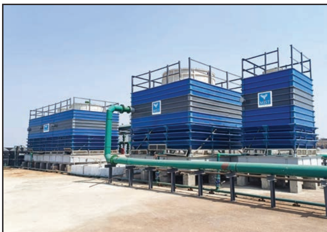
Model-III: Induced Draft Mist Cooling Tower
