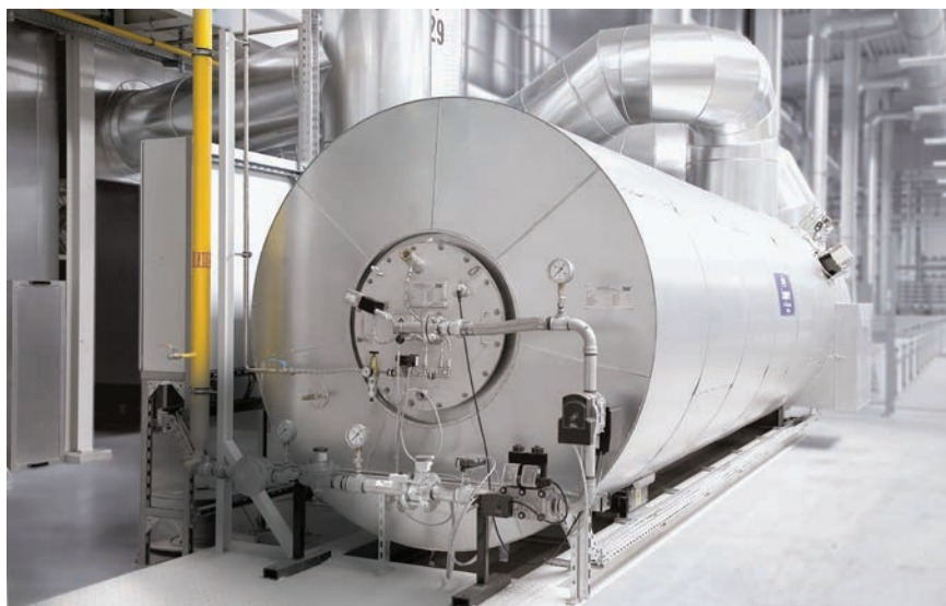
Figure 1: Recuperative thermal oxidizers (Oxi.X.TR)
