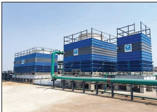
Model-III: Induced Draft Mist Cooling Tower
