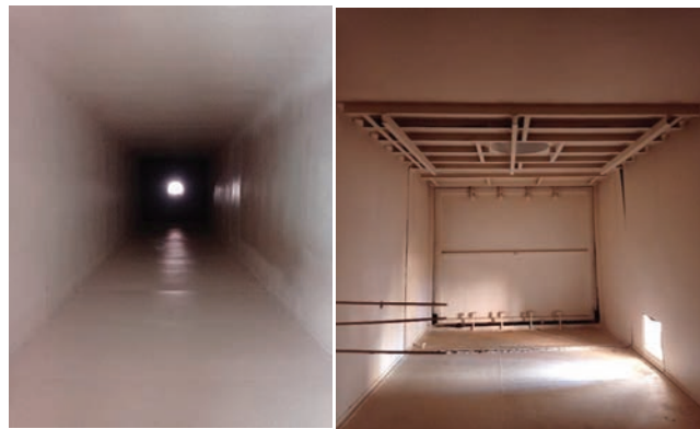
FGD Ducts with Glass Flake Coating for temp upto 200Deg C.
