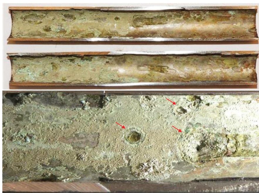
Figure 1: Inner surface of the failed Alloy 400 tubes showing pits and thick greenish scale
