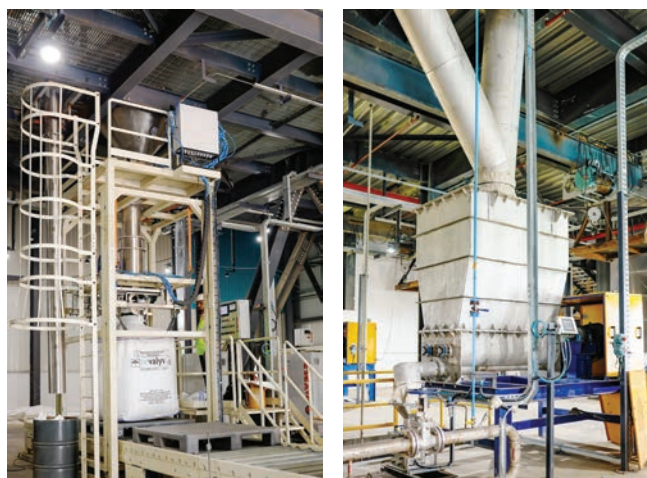
revalyu Resources plant in Nashik, India.
