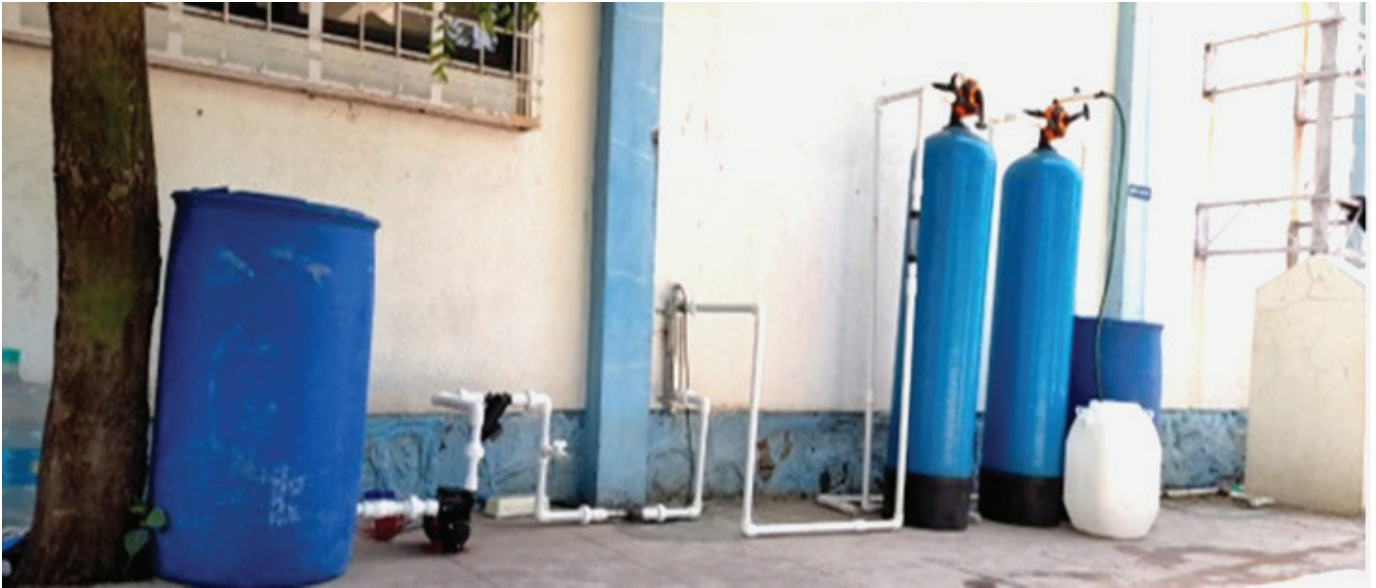
Figure 2: Glass media filtration and AOP technique based tertiary effluent plant for micro-plastics removal (Actual site image)
